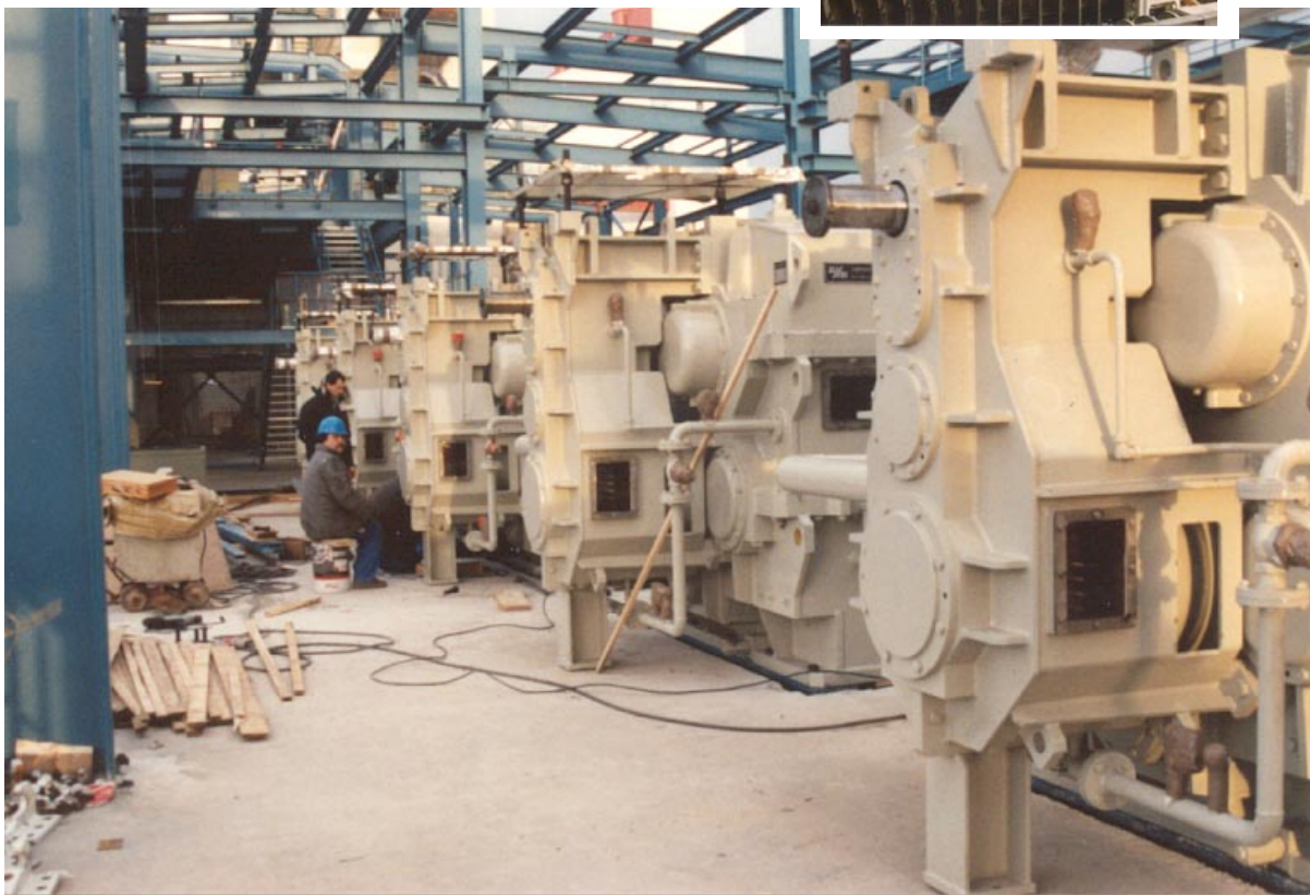
Ja)(Ke-Serviceingenieure bei der Installation der Pressenantriebe Ja)(Ke Service engineers during installation of press drives
